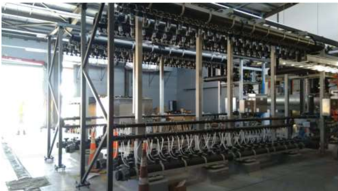
Membrane Hall: Skids ready for the microfiltration membrane units to be installed
