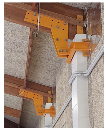
Greerton Seismic brackets
