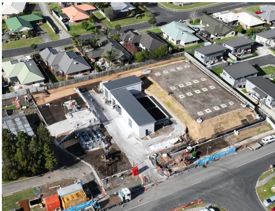
Opal Drive Pump Station
