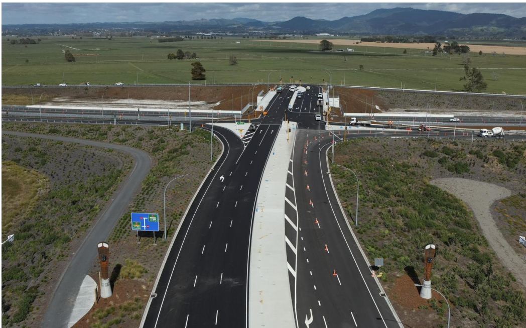
Pāpāmoa East Interchange – aerial perspective from The Sands Ave towards the new overbridge
